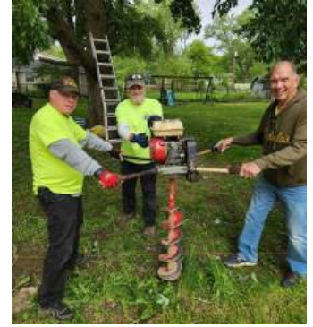
Don Smith, Dave Lothamer, Jim Keefer prepare to drill one of four new post holes.
